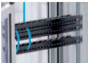
Components for the Floor Distributor
